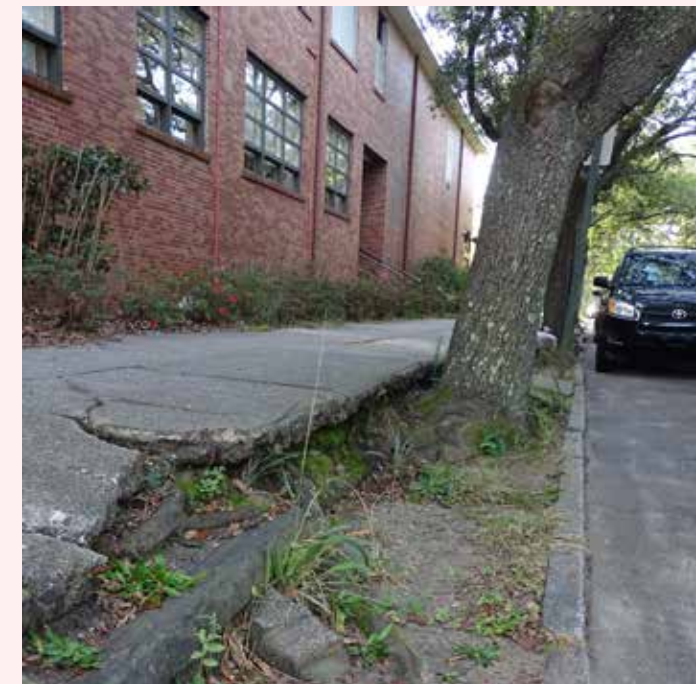
When trees do not have enough room to begin with, they may create their own spaces and cause damage to other infrastructure.
