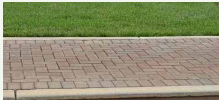
Sidewalks can also be permeable.
