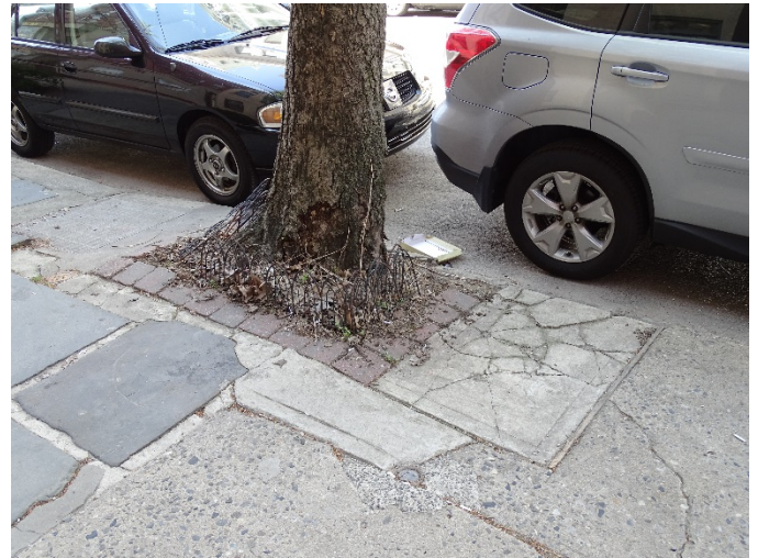
Sidewalk damage from tree roots, causing the need for endless patching.
